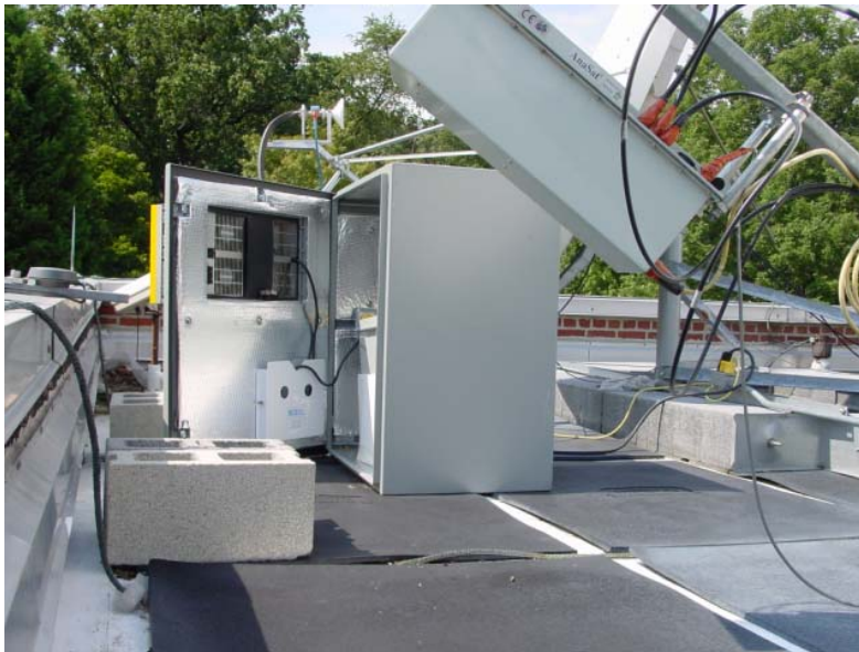
Figure 8. Thermoelectric all-weather chamber for TWSTT electronics.
